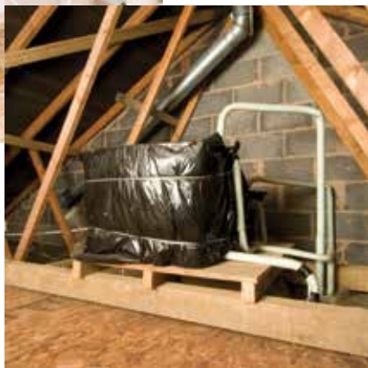
cold water tank installed in the loft
